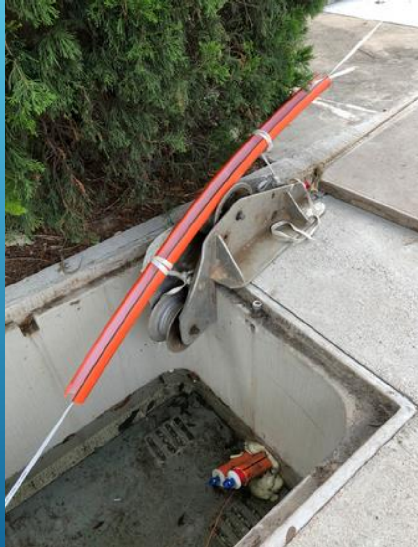
Split Duct Tied to Lip Roller
