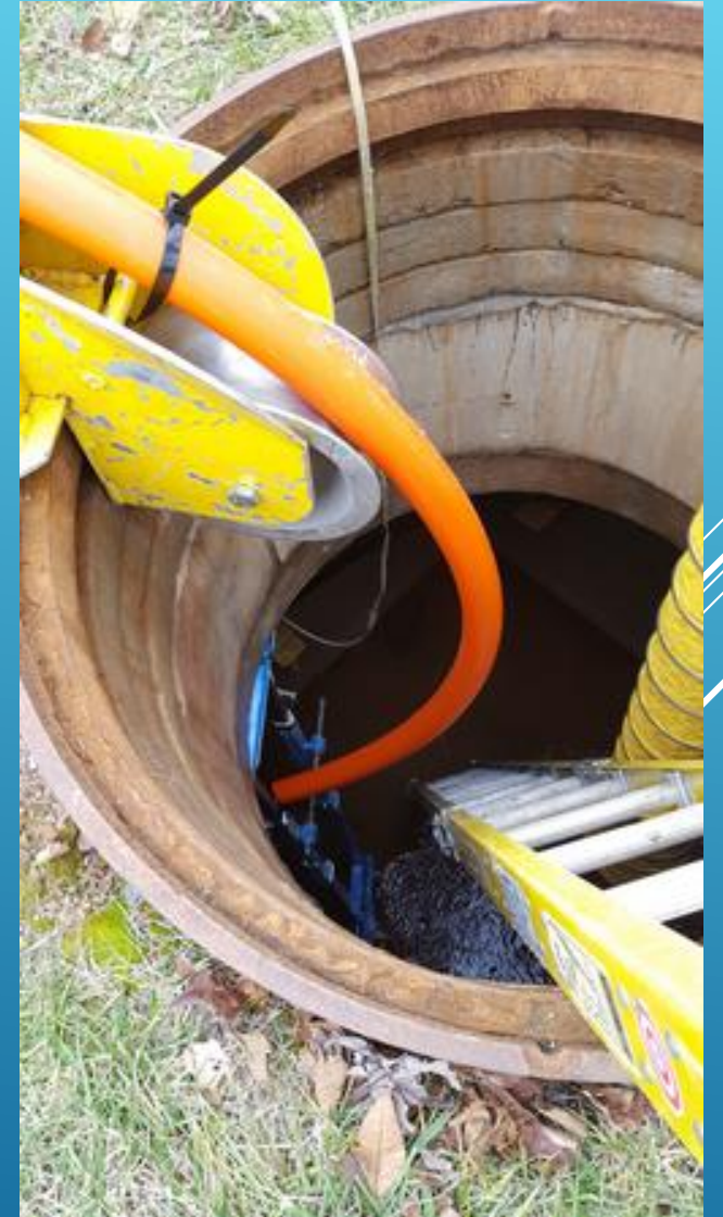
Duct Tied to Lip Roller
